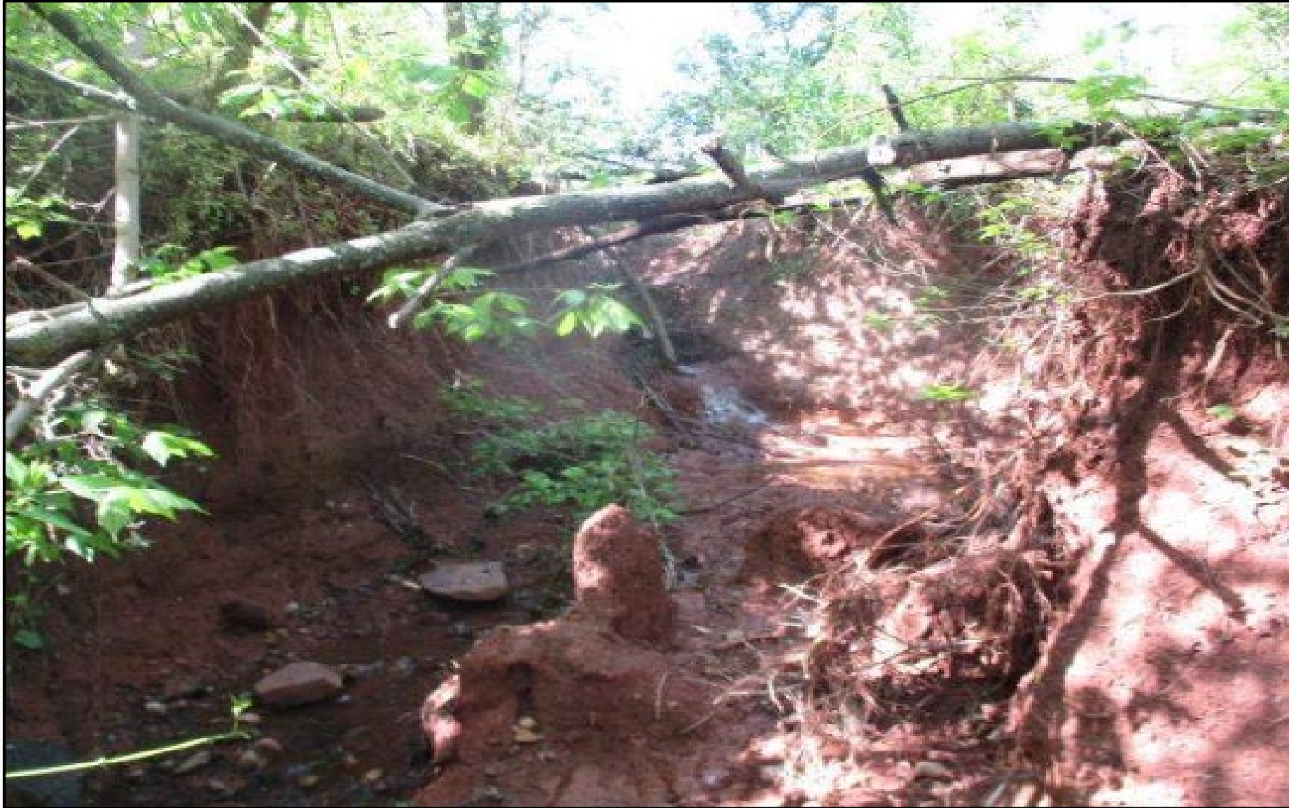
Significant erosion of the emergency spillway receiving channel.
