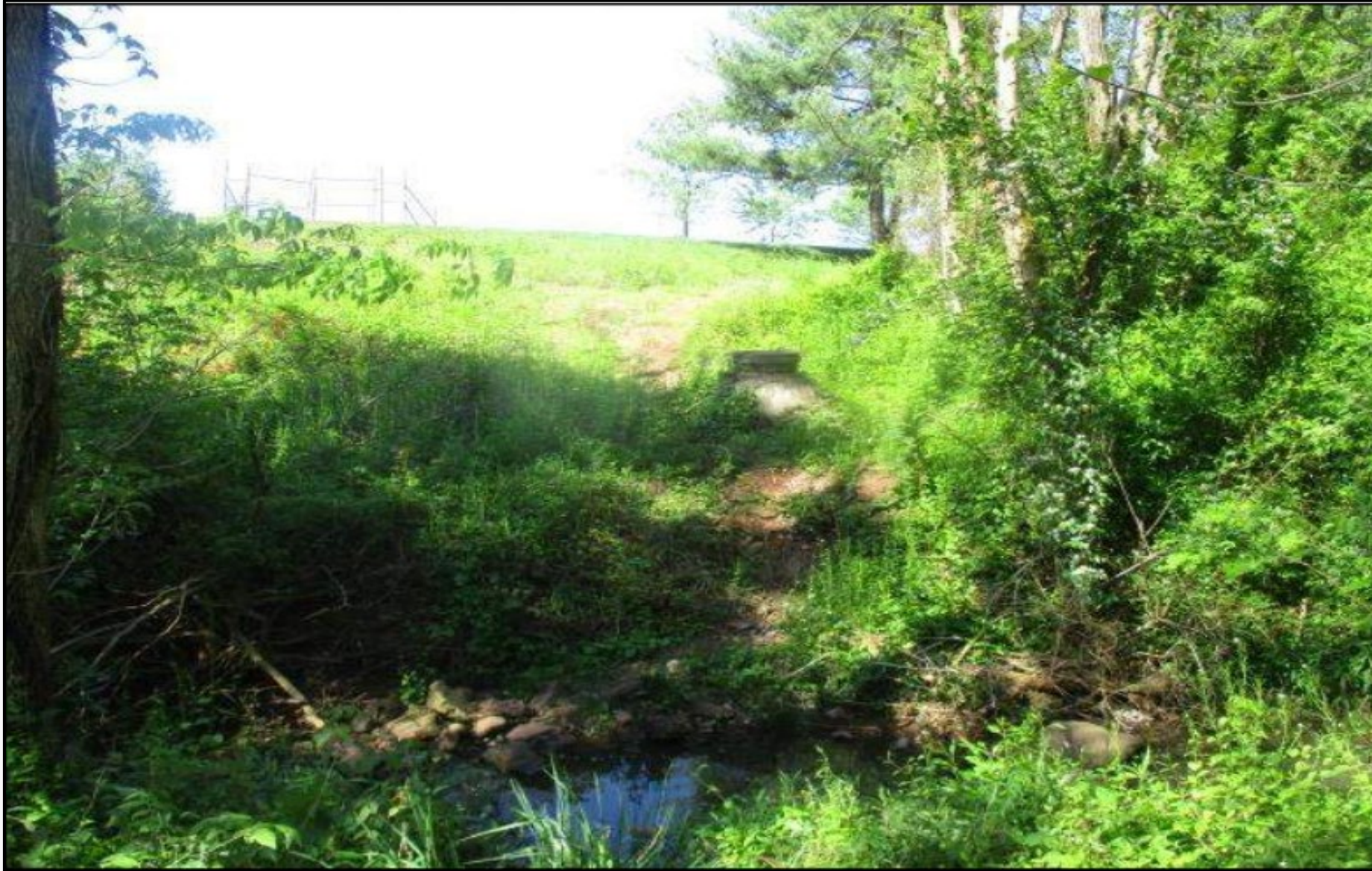
Toe of dam is undercut and eroding.
