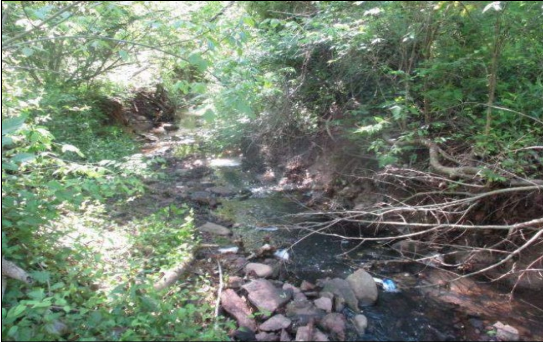
Significant erosion of the principal spillway receiving channel.
